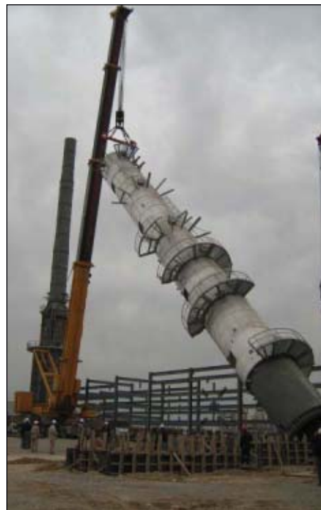
The crude oil distillation tower moves into place at the KAR Oil Refining Ltd. refinery in Iraq.
